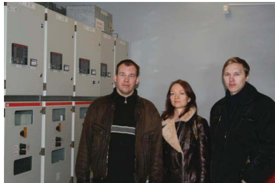
Figure 4. RTU supervisor prof. asoc. A. Ziravecka, Supervisor from industrial partner U. Anitens and student A. Shapovalovs at experimental results monitoring of relay systems Latvenergo division at Jelgava city.
